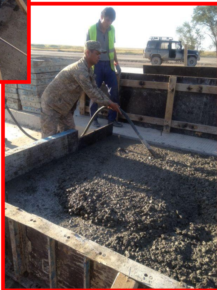
Photo No. 11 : Workers not wearing required protective clothing
